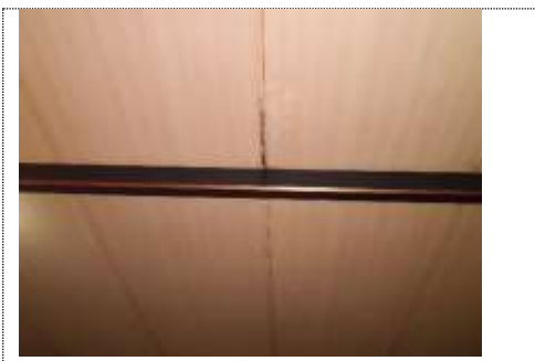
(娯楽室天井 (雨漏り))
